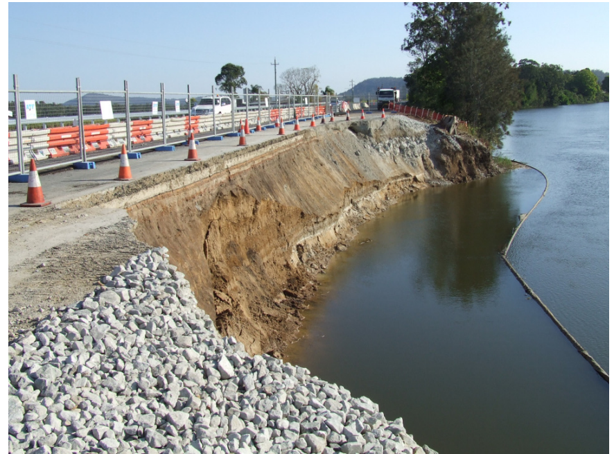
Above: Erosion at Tyndale North, September 2009, courtesy of Scott Lenton, Clarence Valley Council
